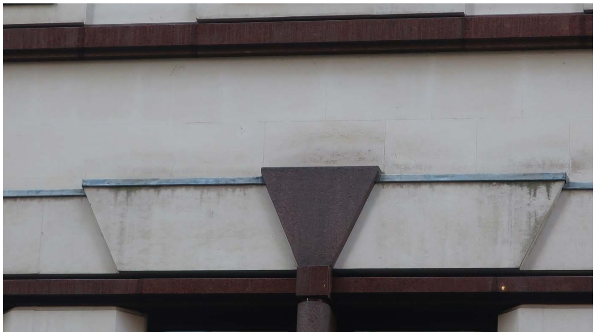
Photograph 14 – Localised damp and algae staining to the original stonework.
