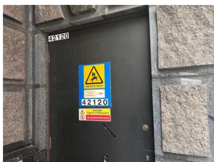
Photo of the substation.
