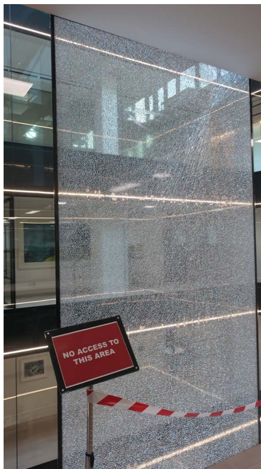
Photograph 22 - Internal atrium wall showing shattered panel at Level 7.
