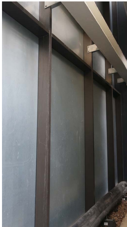
Photograph 20 – The Rockspan composite panels to the plant enclosure are general inaccessible to view.
